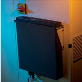
UPS system for tool and machine protection
