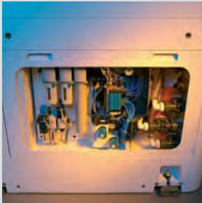
Easy access to utility supply
